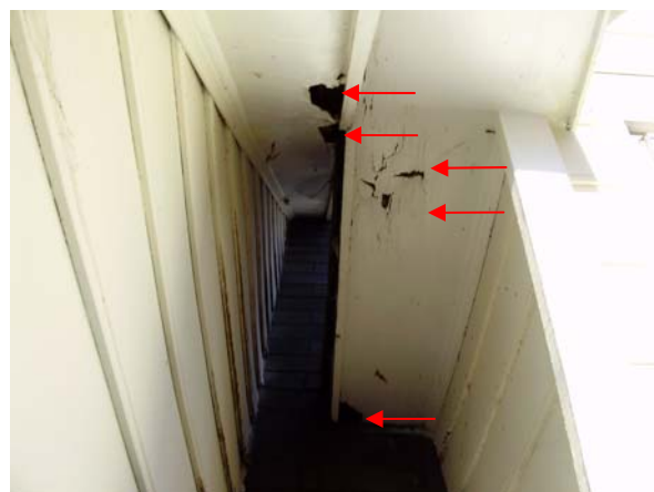
Rodent access holes and moisture damage was noted at the soffit boards on the left side of the left dormer on the front of the home.
