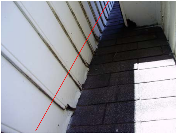
Moisture damage was noted at several pieces of siding along the roofline on the left side of the left dormer on the front of the home.
