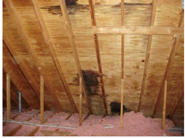
Several stains were present on the plywood roof decking at the rear portion of the attic area above the garage.
