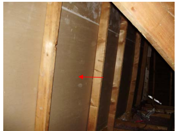
Recommend installing insulation in the left wall of the front, center room in the upper level of the home.
