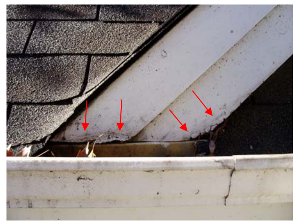
Moisture damage was noted at the fascia boards above the gutter at the bottom of the roof valley above the right wall of the master bedroom.
