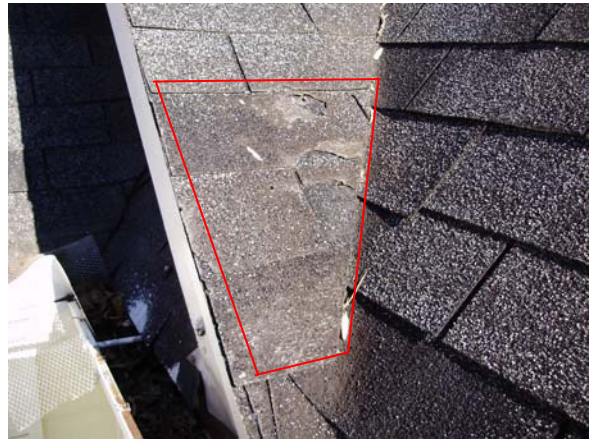
Nail holes and cracks were present in the lower shingles at the bottom of the roof valley above the left wall of the master bathroom.
