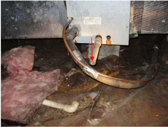
Re-connect the condensate drainline exiting the a/c evaporator coil in the crawlspace.
