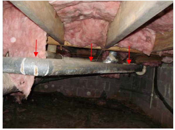
Surface rust was present on the exterior of the main floor furnace flue in the crawlspace.
