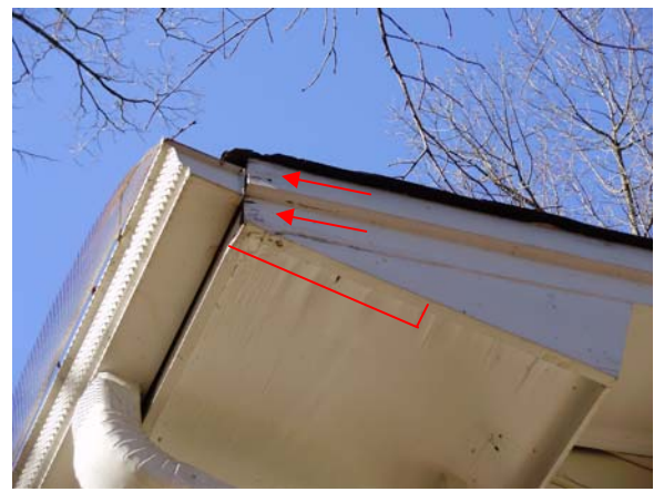
Moisture damage was noted at the fascia/soffit boards behind the gutter at the right corner of the front porch.
