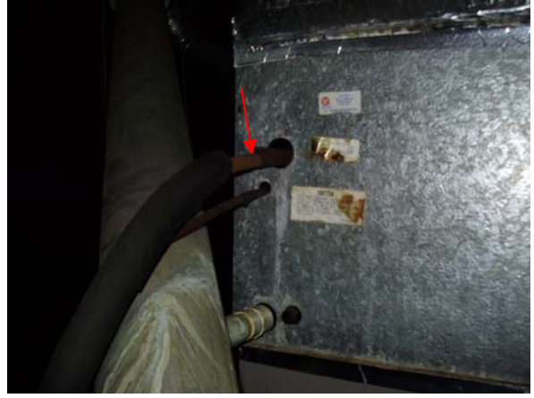
Additional insulation is needed at the voids around the refrigerant return line exiting the a/c evaporator coil in the attic.
