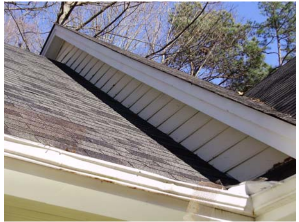
Rodent damage was noted at several pieces of siding along the roofline above the right wall of the garage.
