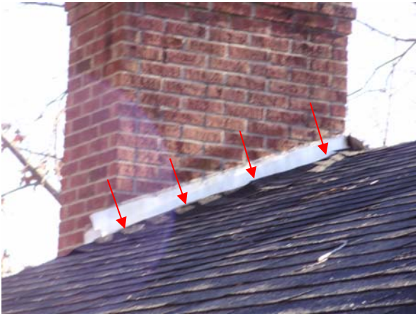
Repair the raised roof flashing along the left side of the chimney chase.
