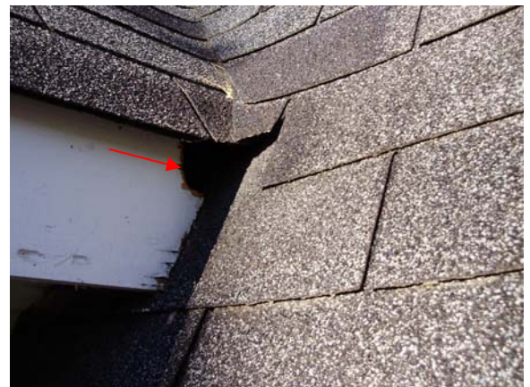
A rodent access hole has been chewed in the rear portion of the fascia board on the right side of the right dormer on the front of the home.
