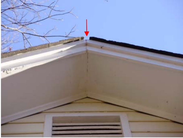
Replace the cracked, outer shingle at the peak of each gable on the home.
