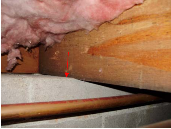
Pressure-treated sill plates were not installed above the foundation walls in the crawlspace.
