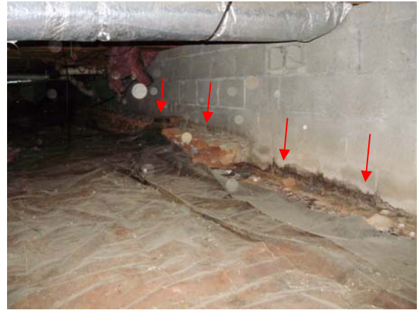
Past moisture stains were present on the lower portion of the rear foundation wall in the crawlspace.
