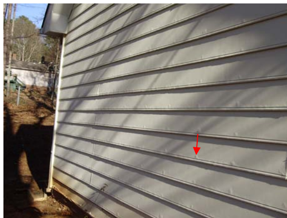
Swelling was present around the nail heads and along the lower edge of various pieces of siding on the left side of the garage.
