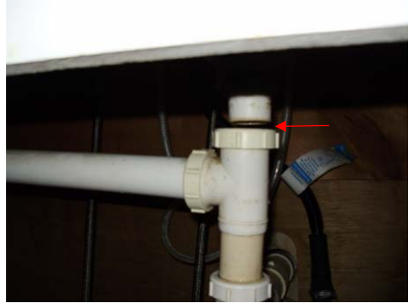
Connect the loose plumbing drainpipe below the right sink in the kitchen.
